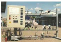
Regulating station SNCR-plant
