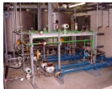
Lime tank with pump and regulating station for two spray absorbers in a waste incineration plant
