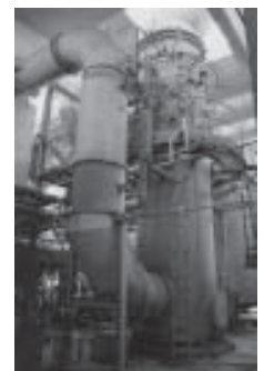
Spray evaporator in an incineration plant for hospital waste
